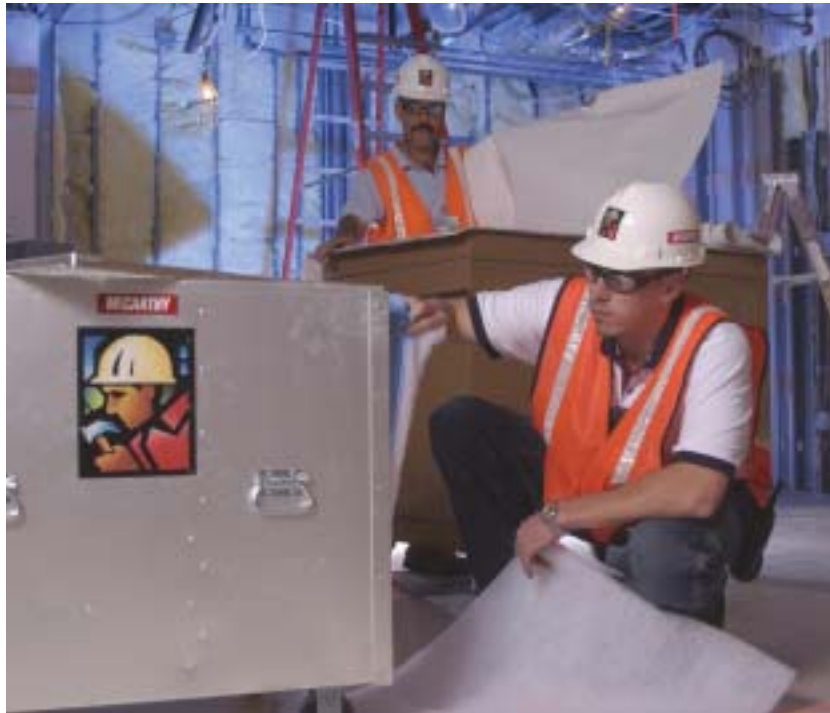
Phil Lafata, Project Engineer with McCarthy, changes one of three screens in the HEPA filter. In the background, Raymond Dauphinais, McCarthy's Project Safety Coordinator, evaluates building plans to determine which air safety measures will be used for the project.
